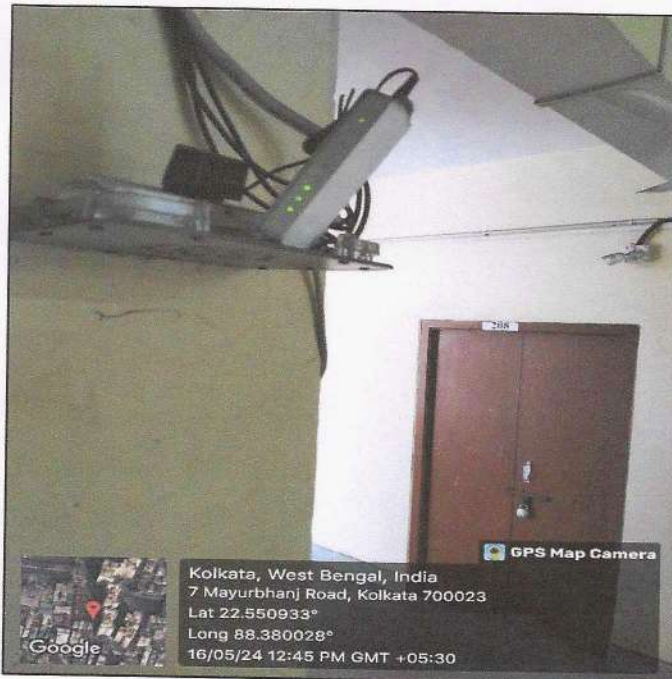
24.4 router at corridor
