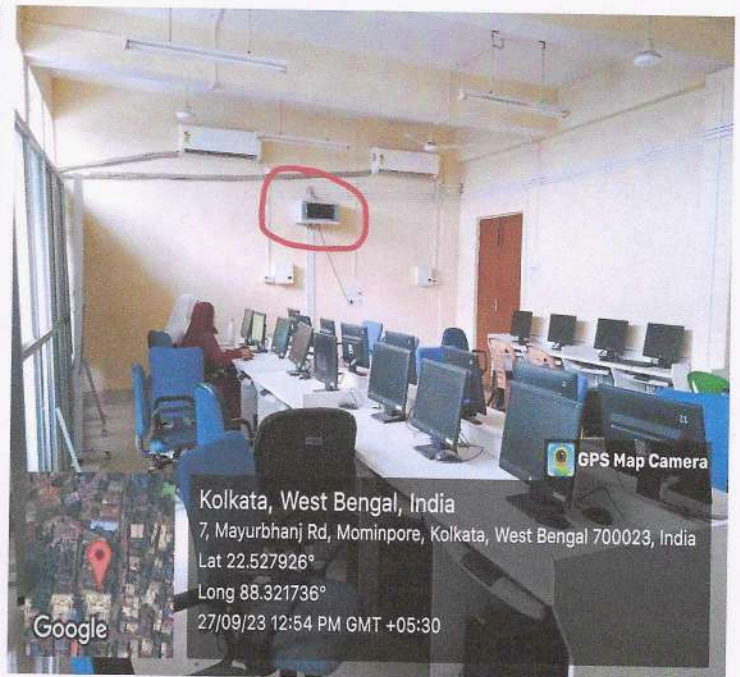
24.5 Internet Connection Distribution box at computer lab
